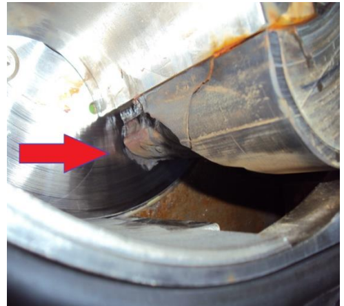
Figure 2: Damaged lobe on pump
